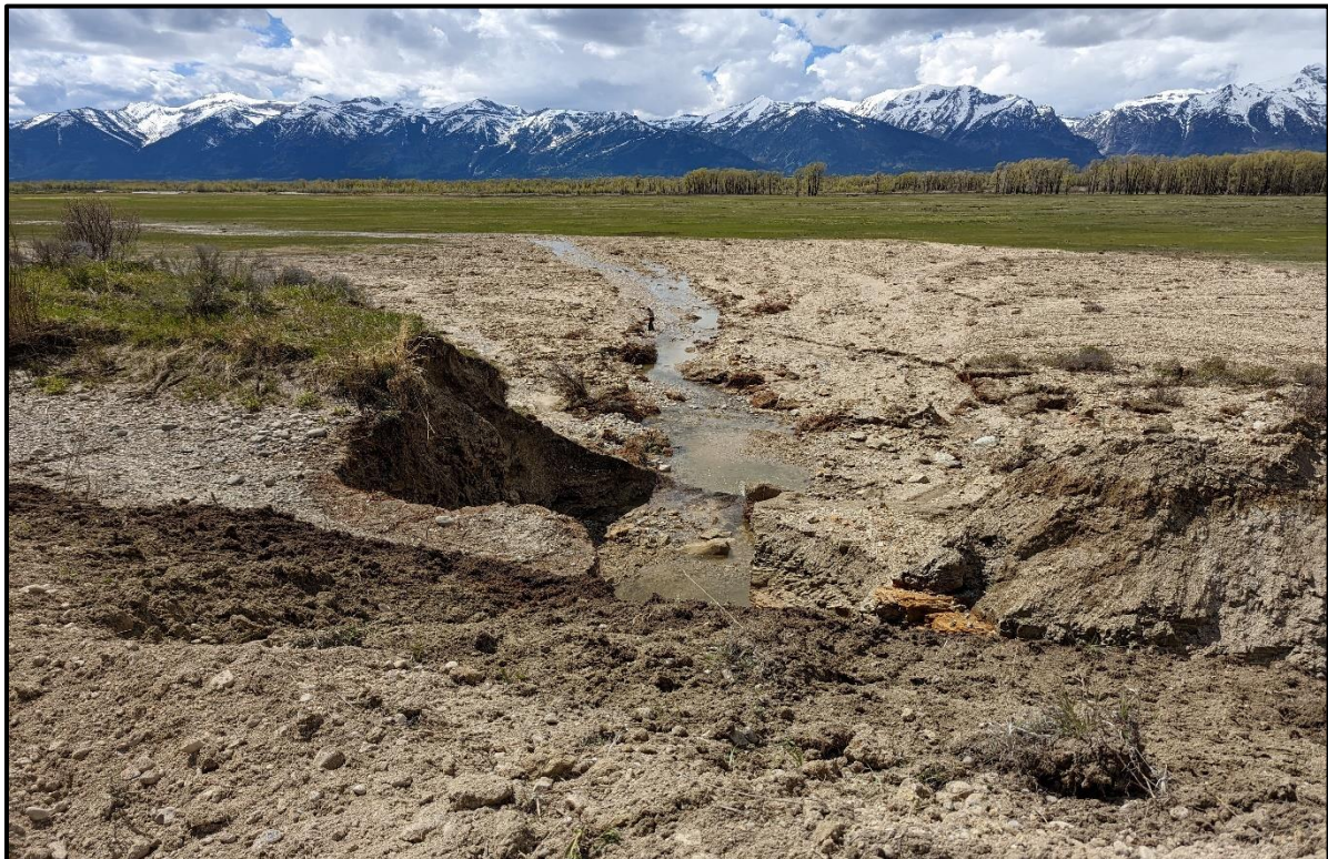
Figure 9: Ditch breach and debris deposition zone. Original/intact section of ditch visible in center left.
