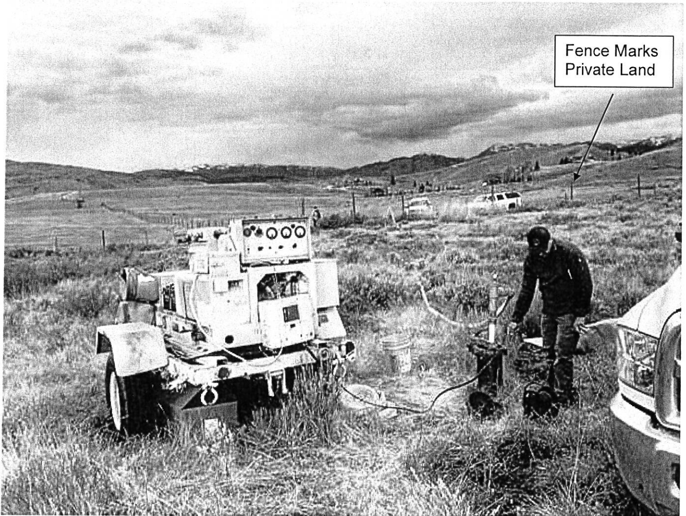
Photo 1. Pump Test Setup on US Forest Land with Generator and Submersible Pump in Well. Discharge Line Running across the Land about 100 feet to Livestock Troughs on Private Land.
