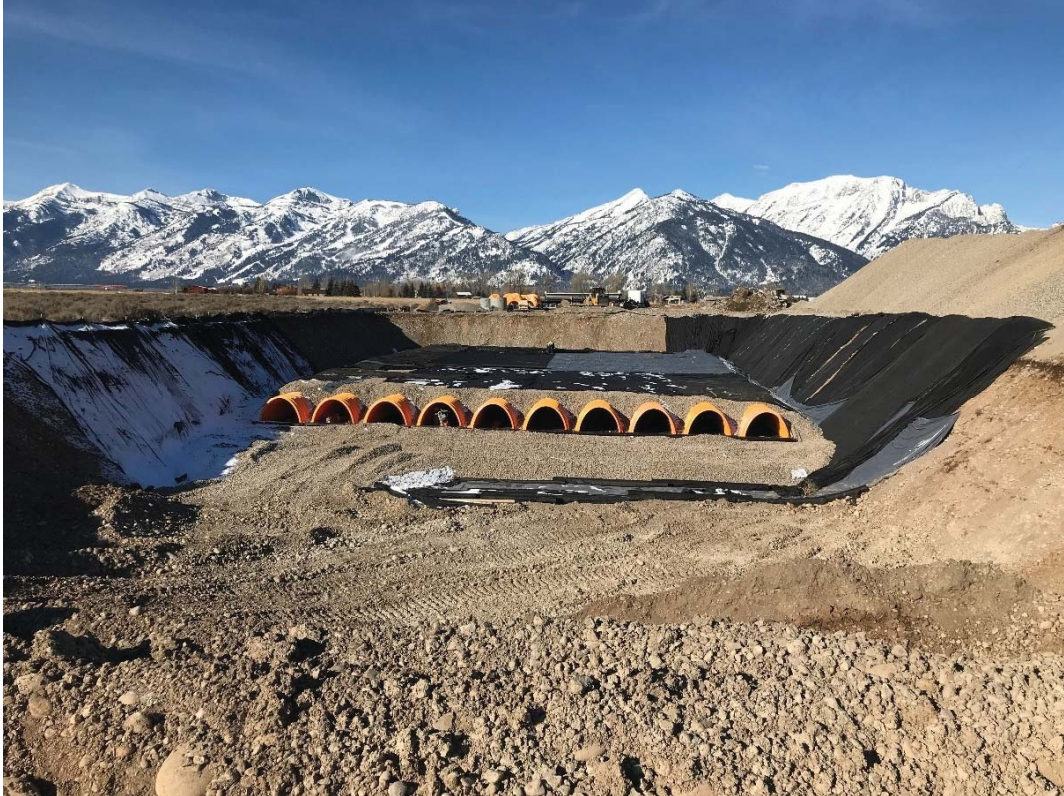
Photo 9: Sub-Contractor installing the top fabric and impermeable liner membrane within the western ¼ of the underground detention and filtration system.
