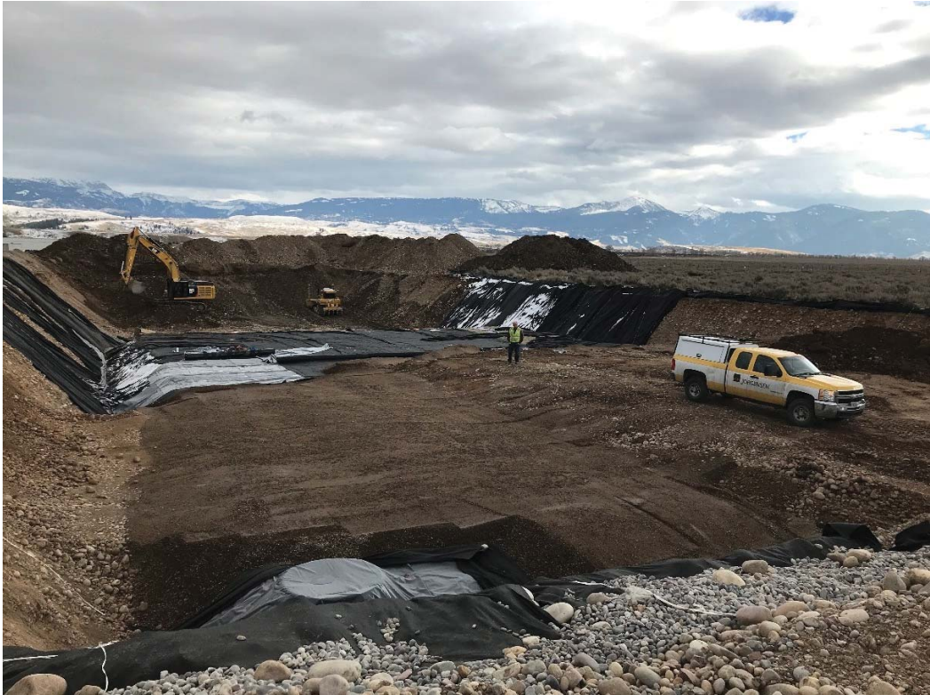
Photo 10: Sub-Contractor installing and compacting native material on top of the system (above the top fabric and impermeable liner membrane) within the western middle ¼ of the system.
